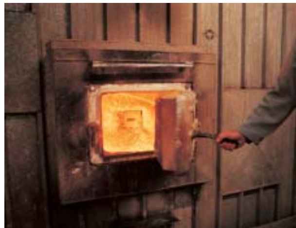
Co-generation plant at Mainz coffee factory, Germany, where spent coffee grounds are used as fuel
